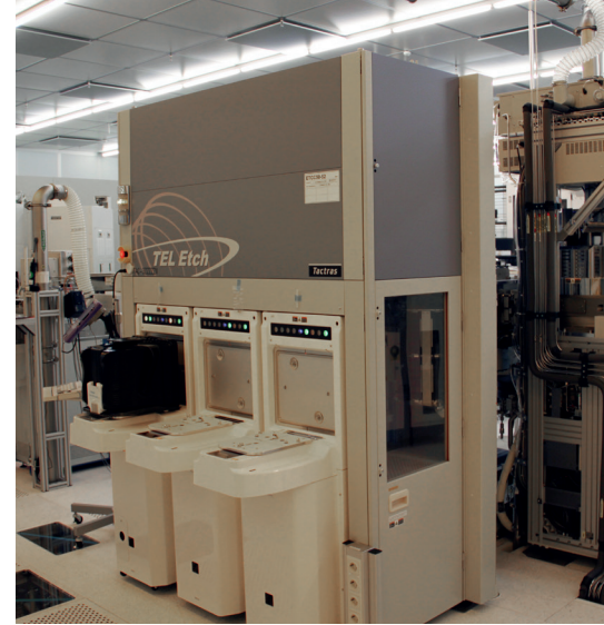
Tokyo Electron Mainframe with VIGUS chamber (specifications see below)
